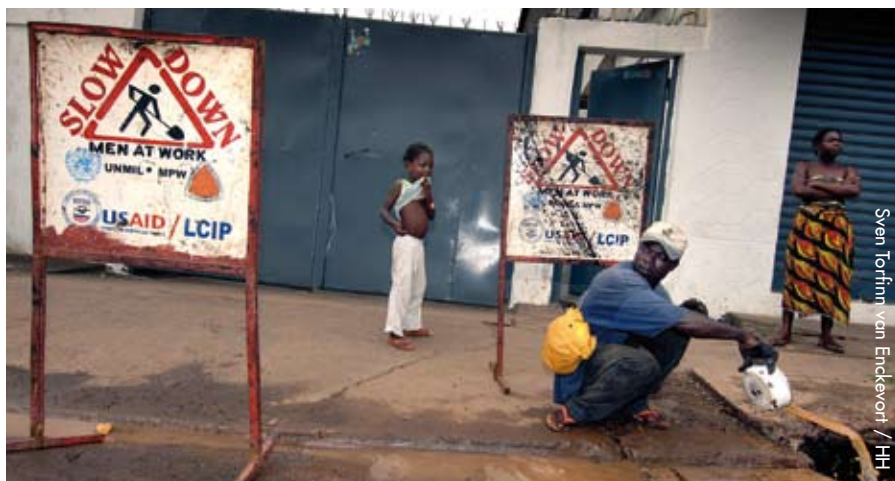
'Operation Pothole': former soldiers and rebels are now employed to repair roads in Monrovia.
